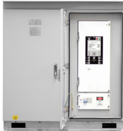
CONTROL AND COMMUNICATIONS CUBICLE
