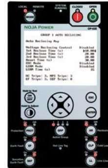
PANEL DE CONTROL LOCAL
